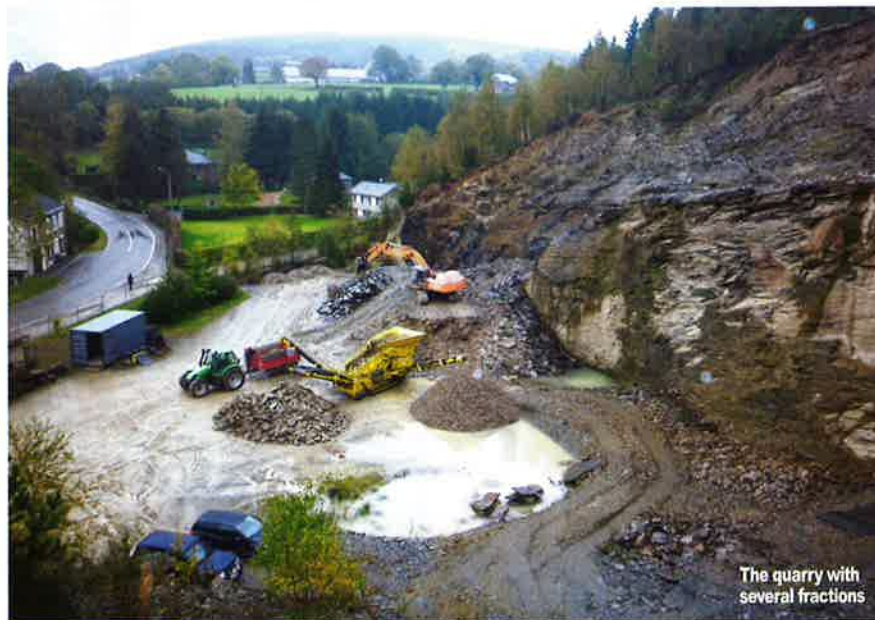
A two-day test of the Keestrack Combo was carried out in the quarry
